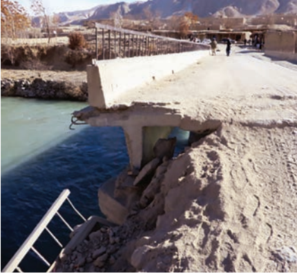
Structural damage to a CERP-funded bridge in Baghlan Province. (SIGAR photo)
