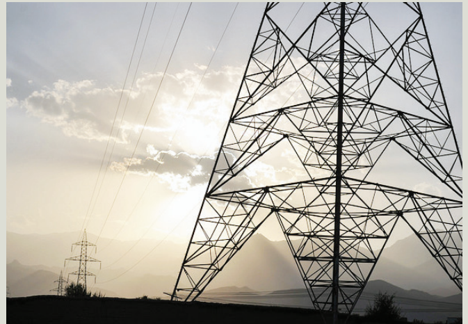
Power pylons on the outskirts of Kabul. (Asian Development Bank photo)
